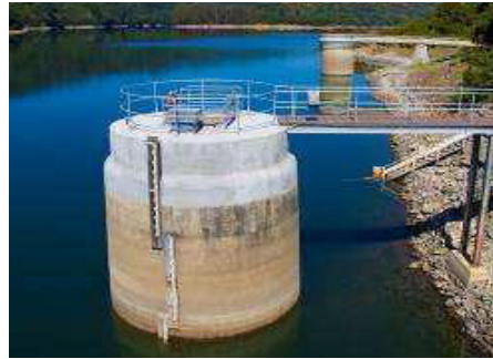
After upgrading, this part of the Crystal Spring Dam's outlet structure will be submerged and no longer visible.
